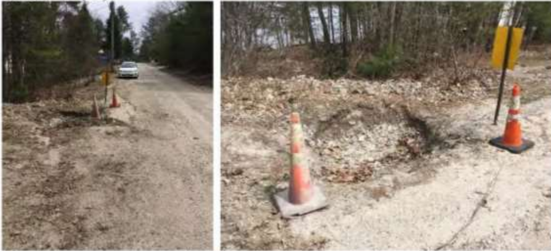
Sloped road approaching site (left), eroded hole at clogged culvert outlet (right).
