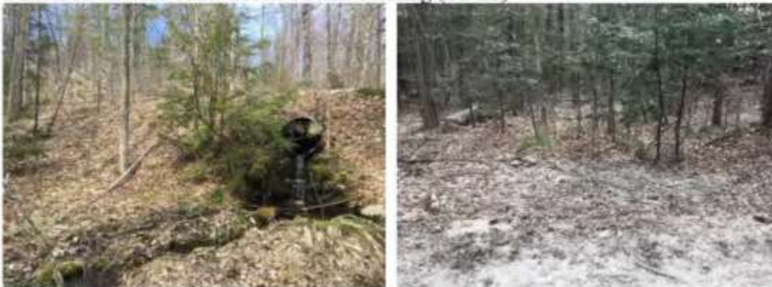
Culvert outlet from downstream (left), sediment washing down bank to right of culvert (right).
