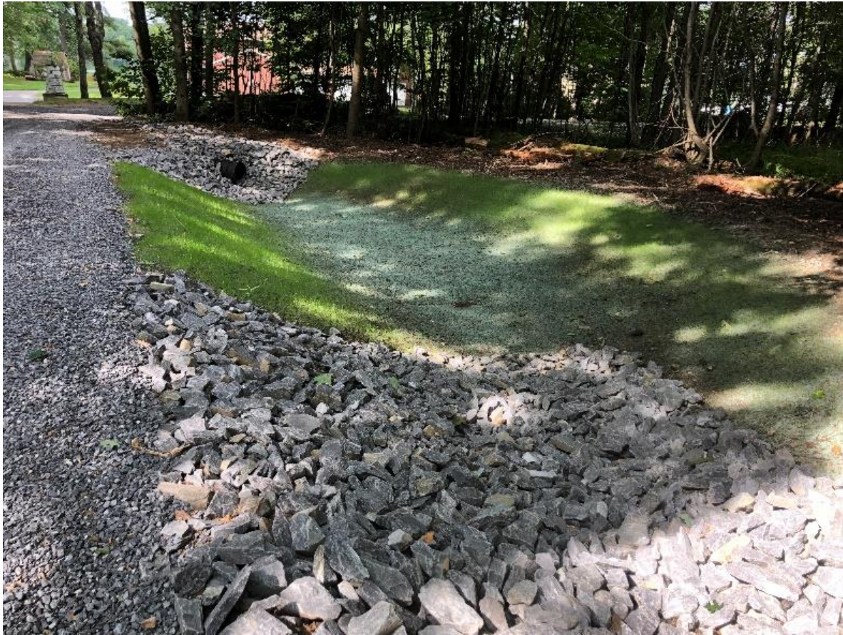
Watchic Road 3. Small retention pond / raingarden installed over crushed stone and loam, currently seeded with grass. Blueberries, ferns, and other native plant to be added in the fall
